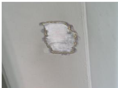
Below: Close-up. The thickness of the coating is quite visible.
