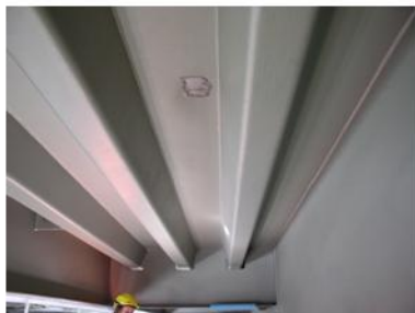
Above: Test is done. Note: The thickness of the coating is approx. 1500 microns!
